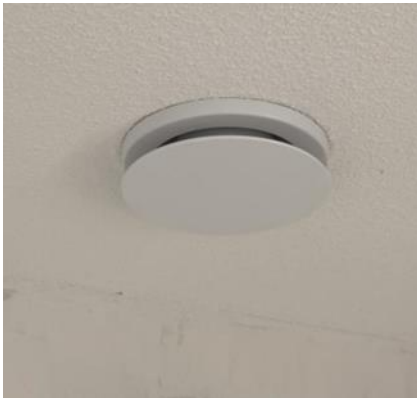
Regulating the extraction valve
