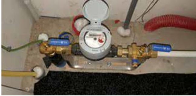
The water pipe is open.
